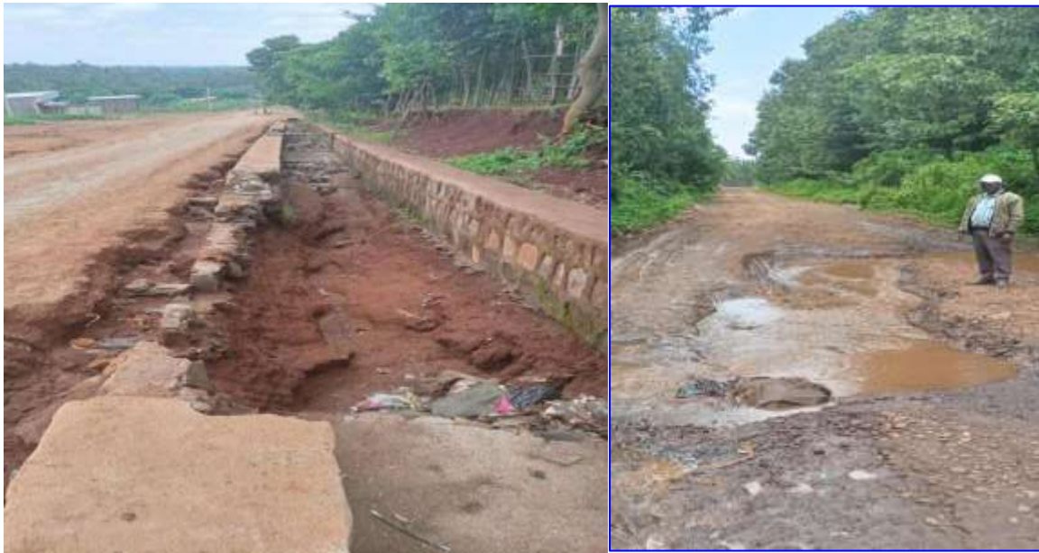
Fig.4: Road condition survey of Boditi to Badessa
